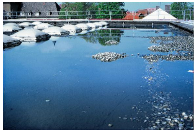
Flat roof construction with standing water. This construction will eventually fail
