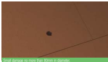
Small damage no more than 80mm in diameter.
